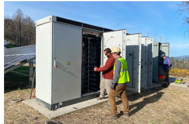
Example of a Containerized BESS Unit
