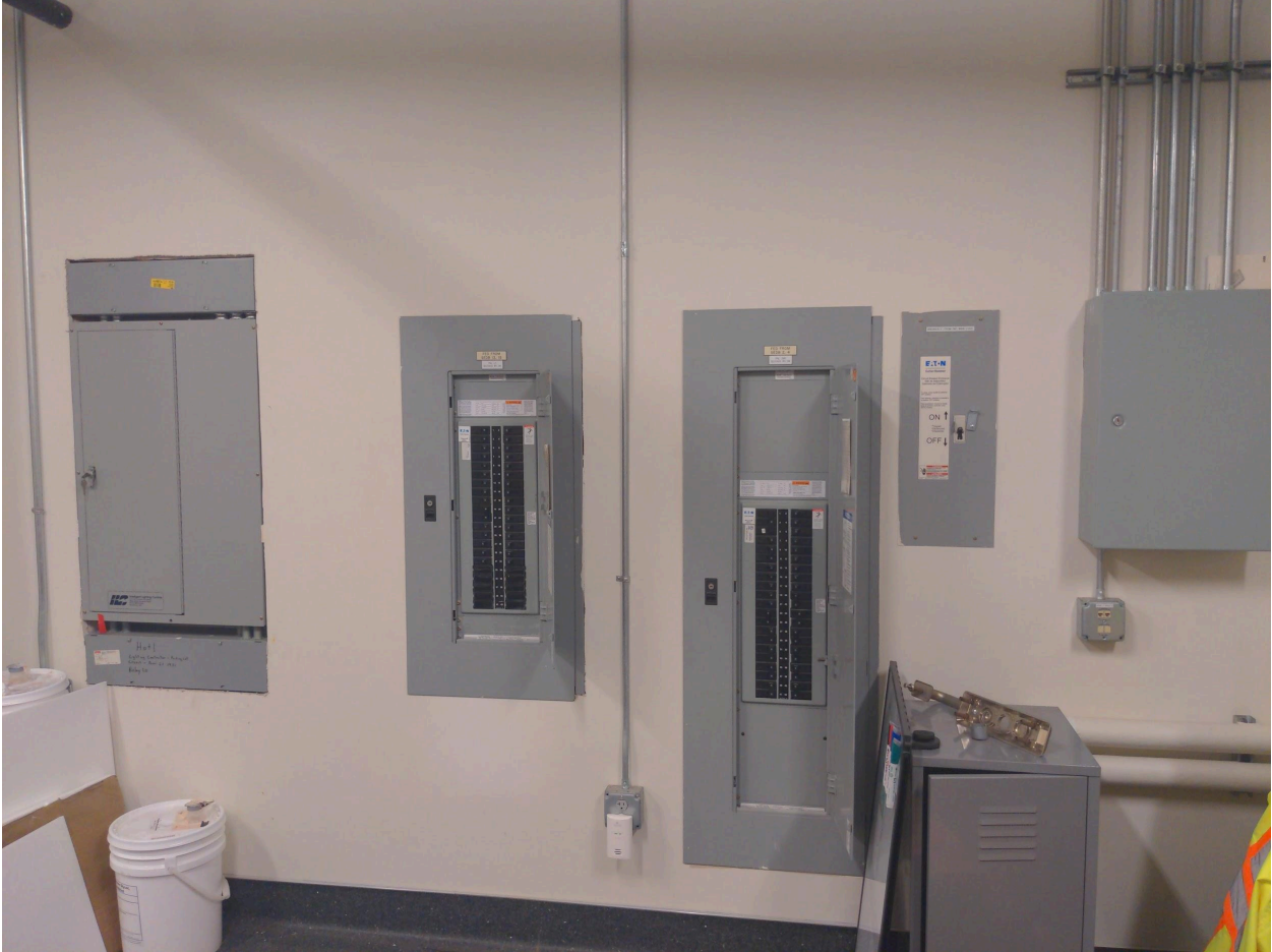
Sub Panel 2M1 and L1 w/Surrounding Equipment:
