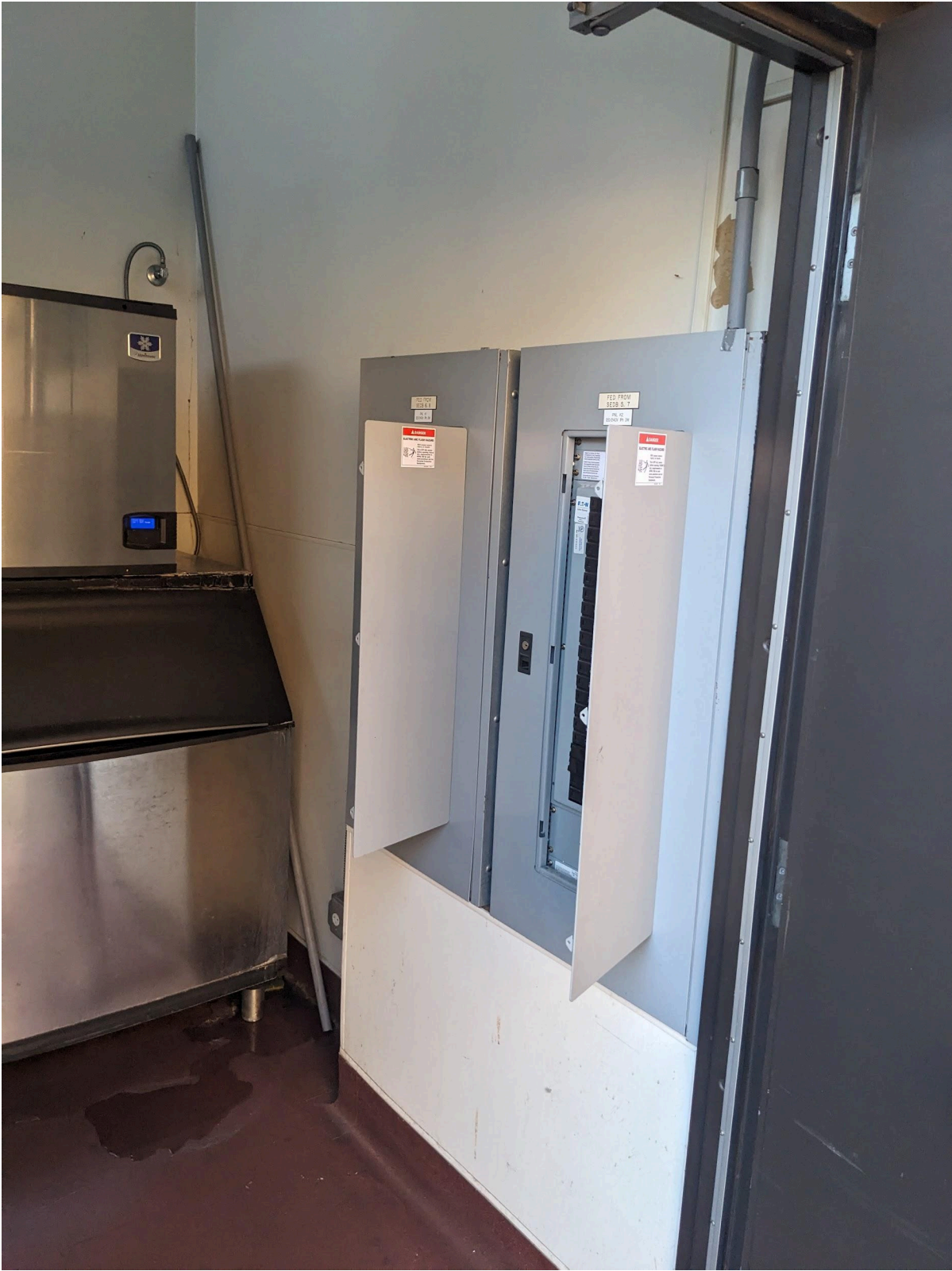
Sub Panel K1 and K2 w/Surrounding Equipment:
