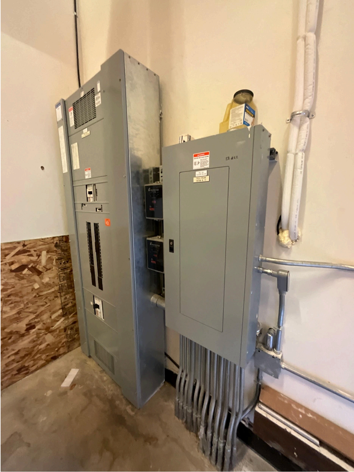
Sub Panel 2P1 w/Surrounding Equipment:
