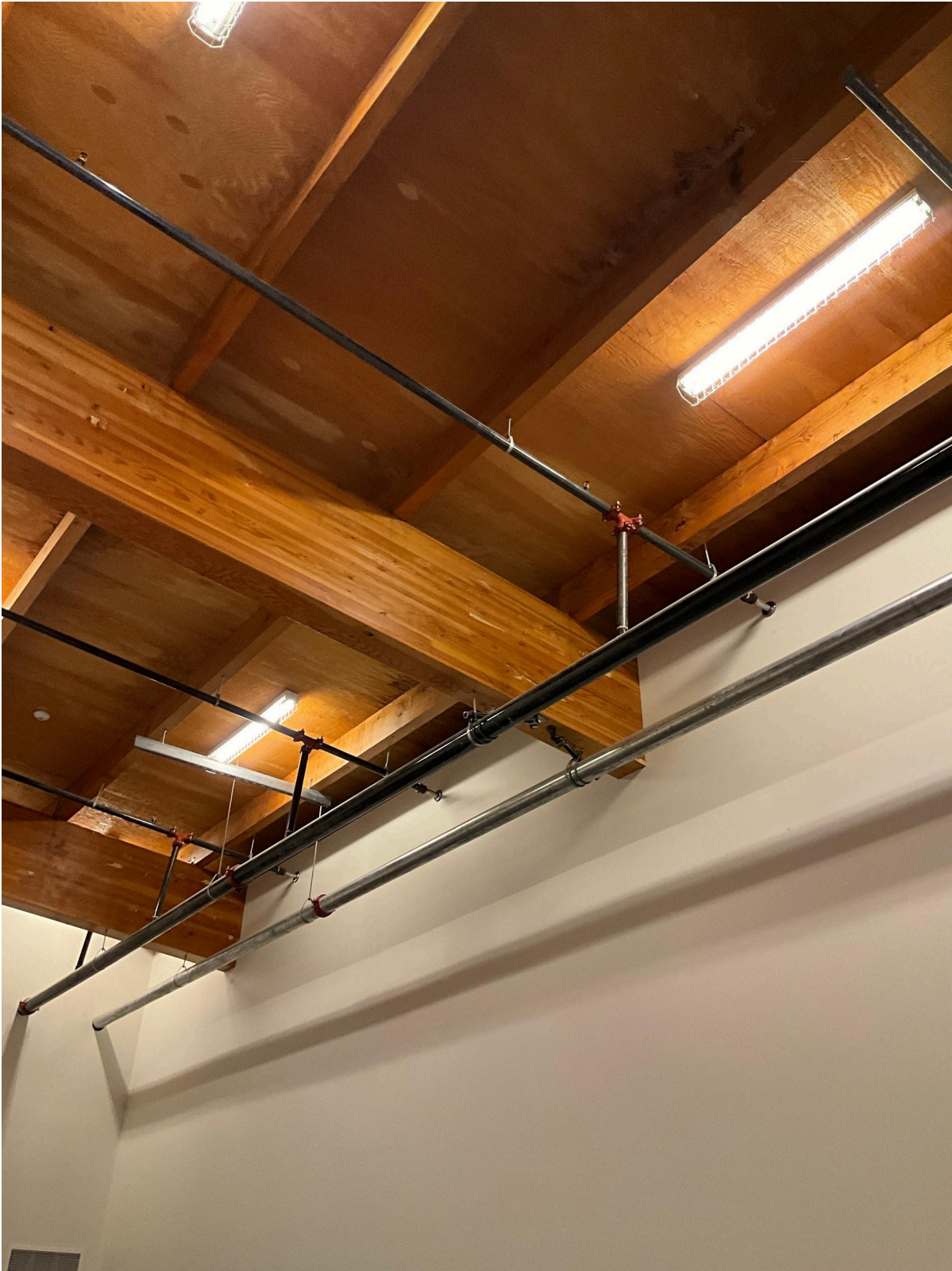
Interior Sprinkler Photos (Minimizes Fire Setbacks per 2015 IBC):
