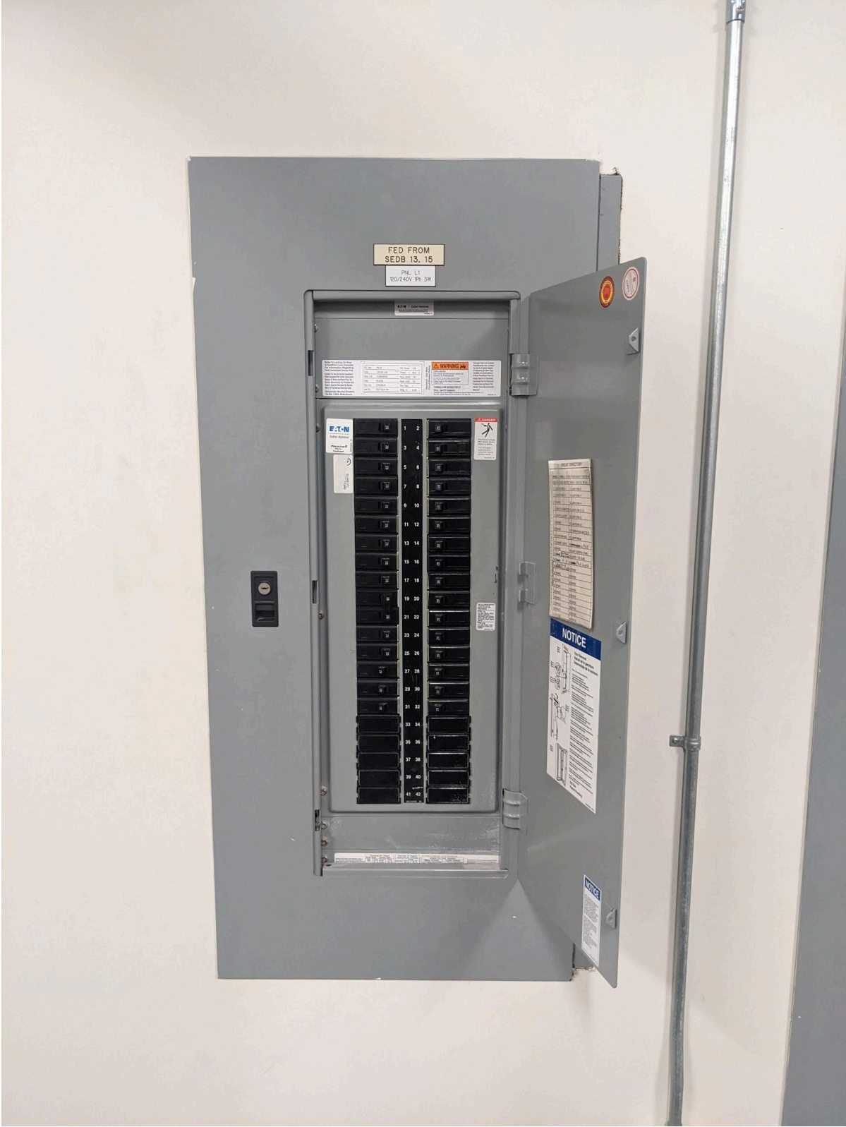
Sub Panel L1 Breaker Close-up/Detail:
