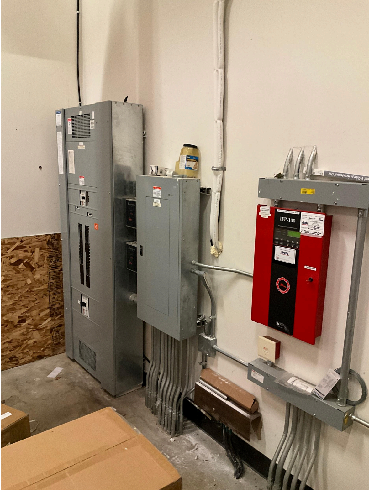
Main Distribution Panel w/Surrounding Equipment:
